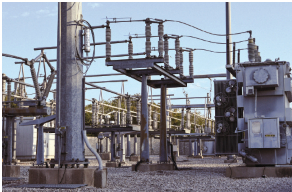
An Austin Energy substation in East Austin
