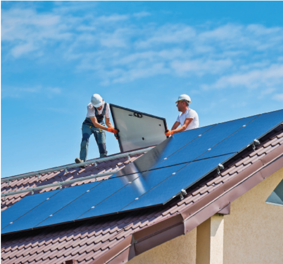
Funding will support solar infrastructure in Austin
