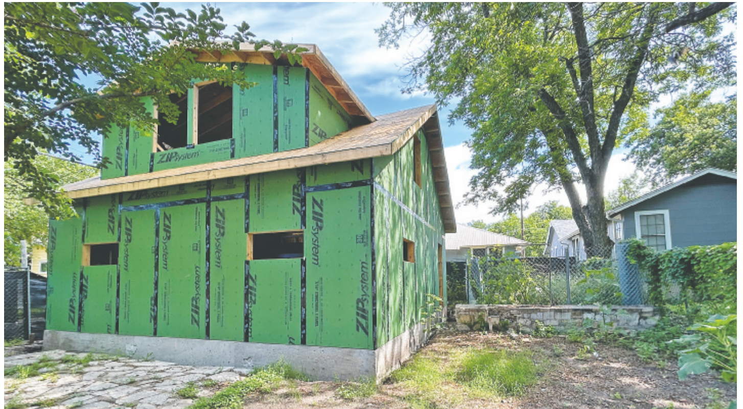
A new, relatively small home goes up in a backyard in North Austin
