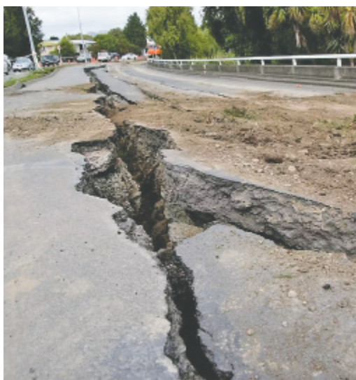
A road in Turkey is cracked down the middle after a 7.8 magnitude earthquake hit the country on Feb. 6
